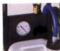
Suction pressure and operation check
